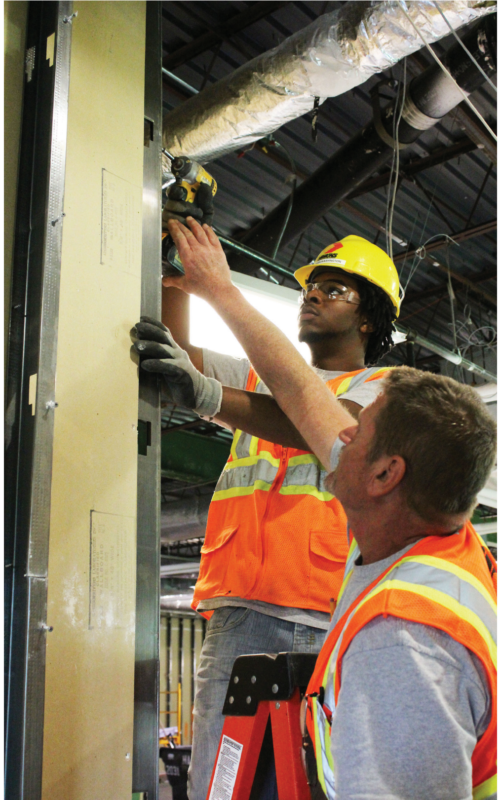
ON THE JOB. Keven Washington, Jr., an Omaha North graduate, gets some guidance from Mark Weatherbee, a Hawkins Construction site supervisor. Weatherbee is supervising the interior demolition of a building on the Bellevue University campus. Washington, who discovered his career interest while exploring trades in the Avenue Scholars program, started working for Hawkins Construction May 9.
